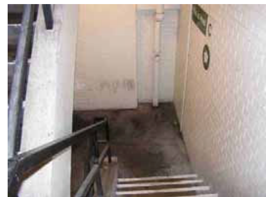
Photo 7: Non-refurbished stairwells at multi storeys
